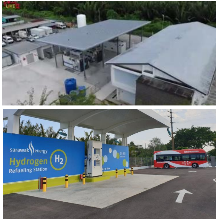
Figure 3.28. Sarawak Energy's Hydrogen Production Plant and Hydrogen Bus Terminal
