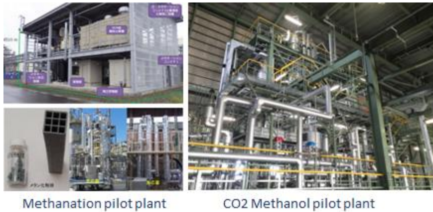
Figure 2.20. Pilot Plant of Methane and Methanol Syntheses from CO 2
