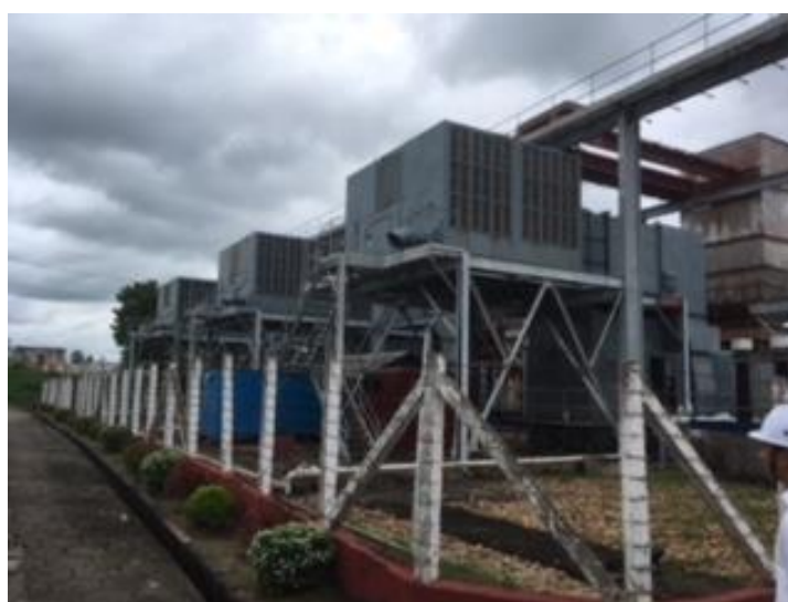
Figure 6.3: Shwedaung Gas-Turbine Power Plant
