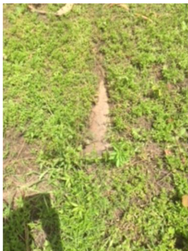
Figure 6.6: Unprotected Pipeline Appearing Aboveground at Aung Lan Bar Station
