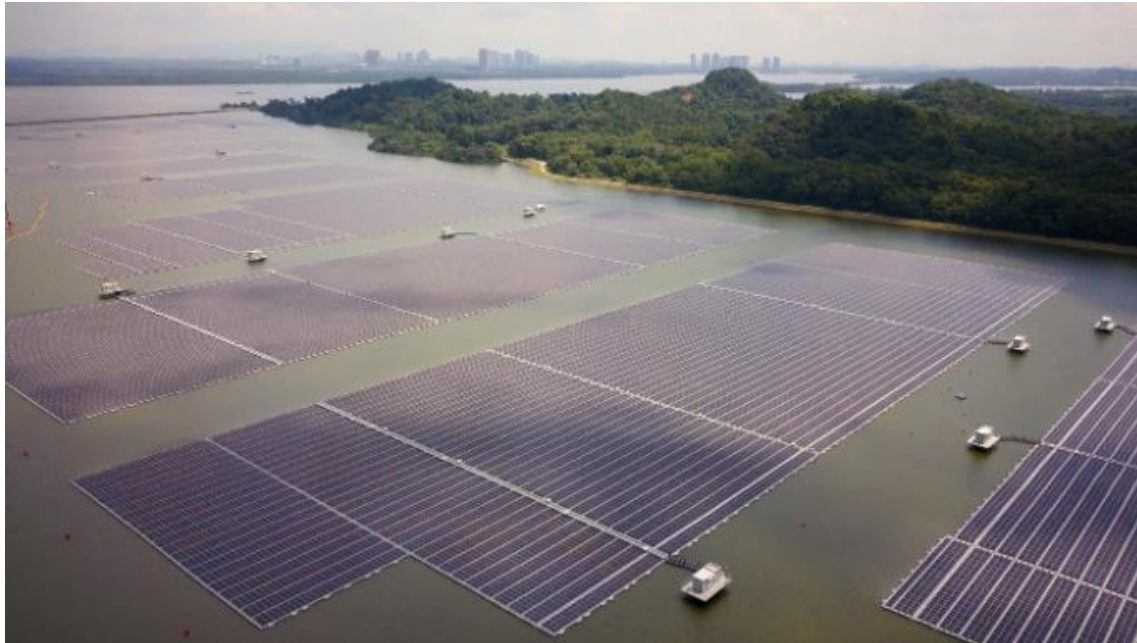
Figure 2.2. Tengeh Floating Solar Farm in Singapore
