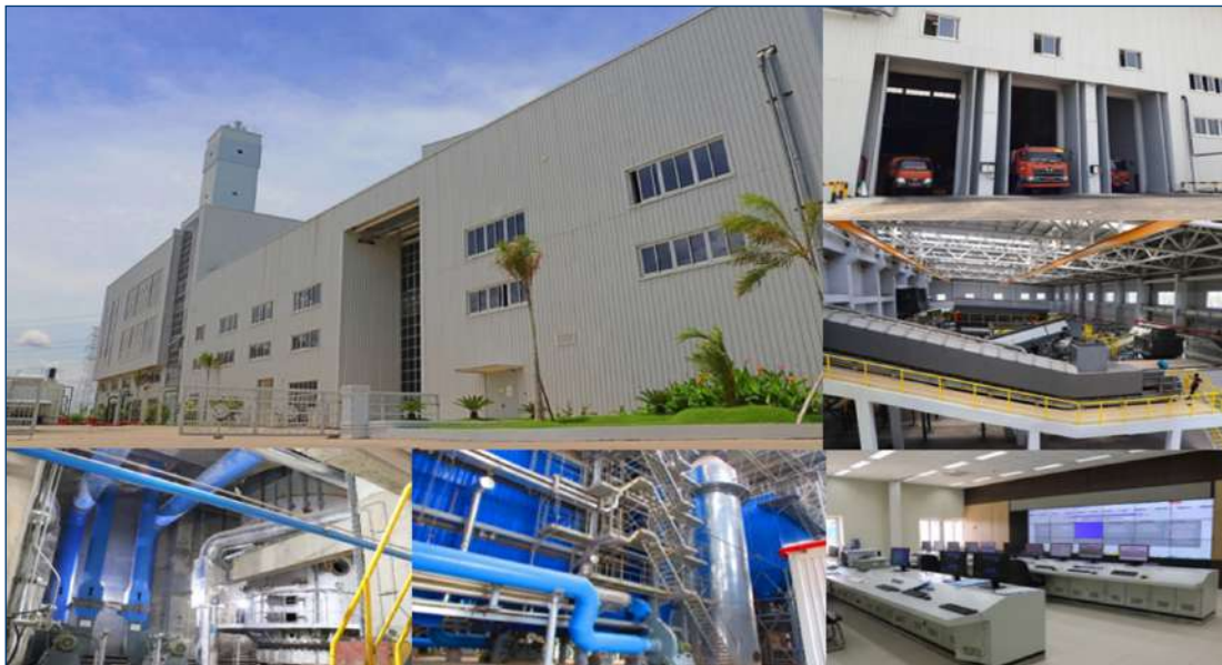
Figure 3.87. Gasification Power Plant at the Benowo WTE Plant
